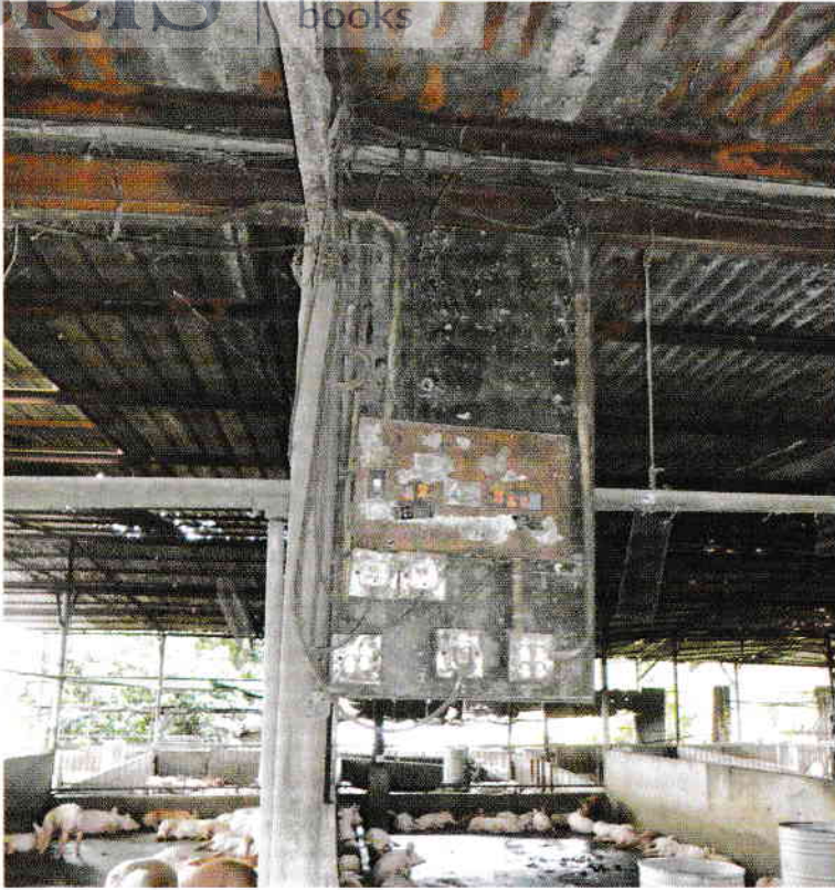
Fig. 1.4ii. Electrical box for wires and fuses in an open area of the pig farm.
