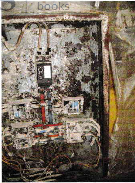
Fig. 1.2ii. Damaged farm-building electrical system.
